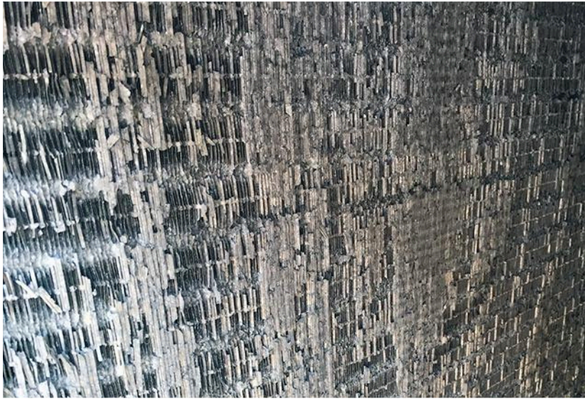
Coil corrosion can create formicary and pitting processes that ultimately lead to leaks.
