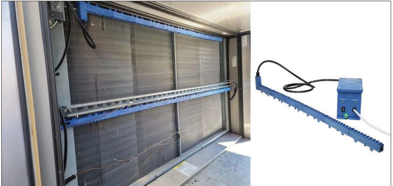
Figure 4. Needlepoint Bipolar Ionization installed on upstream side of cooling coil to reduce microbial growth
