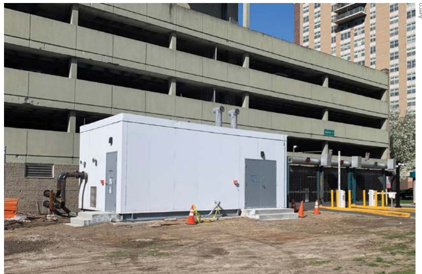
Each of the eight EnviroSep modular plants services a mechanical room in an adjacent parking garage surrounded by a cluster of high-rises.
