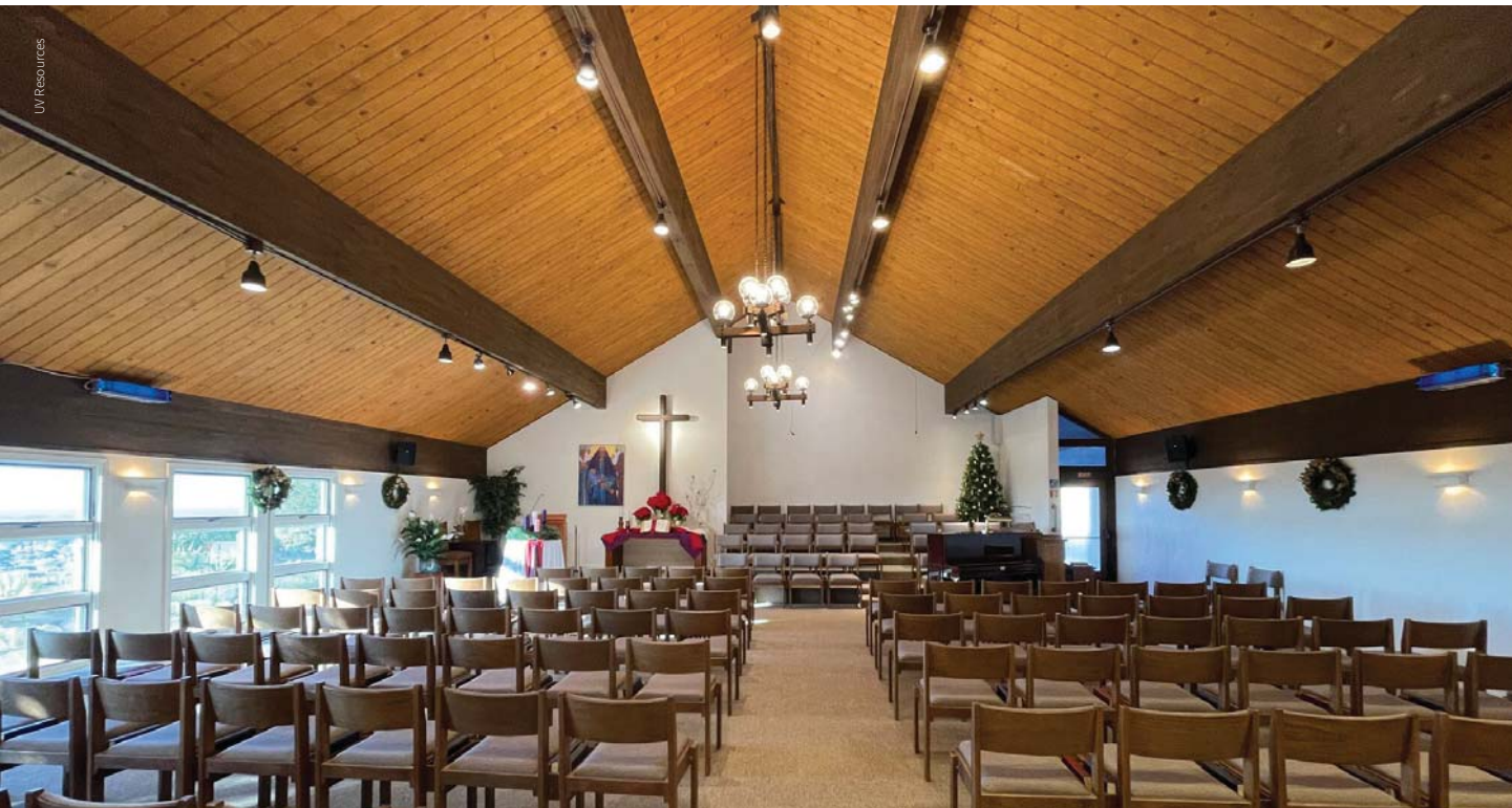
Two GLO-225 baffled or louvered-type luminary units were mounted above occupants’ heads on either side of the sanctuary.
