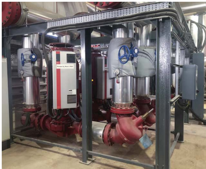
An intelligent packaged pumping system provided in support of a district heating installation in Amiens, France. This network serves more than 19,000 apartments and more than 90% of the city's commercial buildings.
